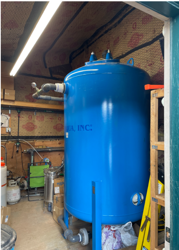
NEW PLUMBED SAND FILTER, RATED 60 YRS +
